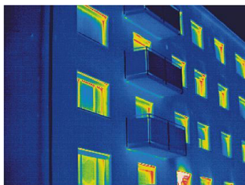
Thermography before and after retrofitting: the more blue colour, the better the insulation of the building
